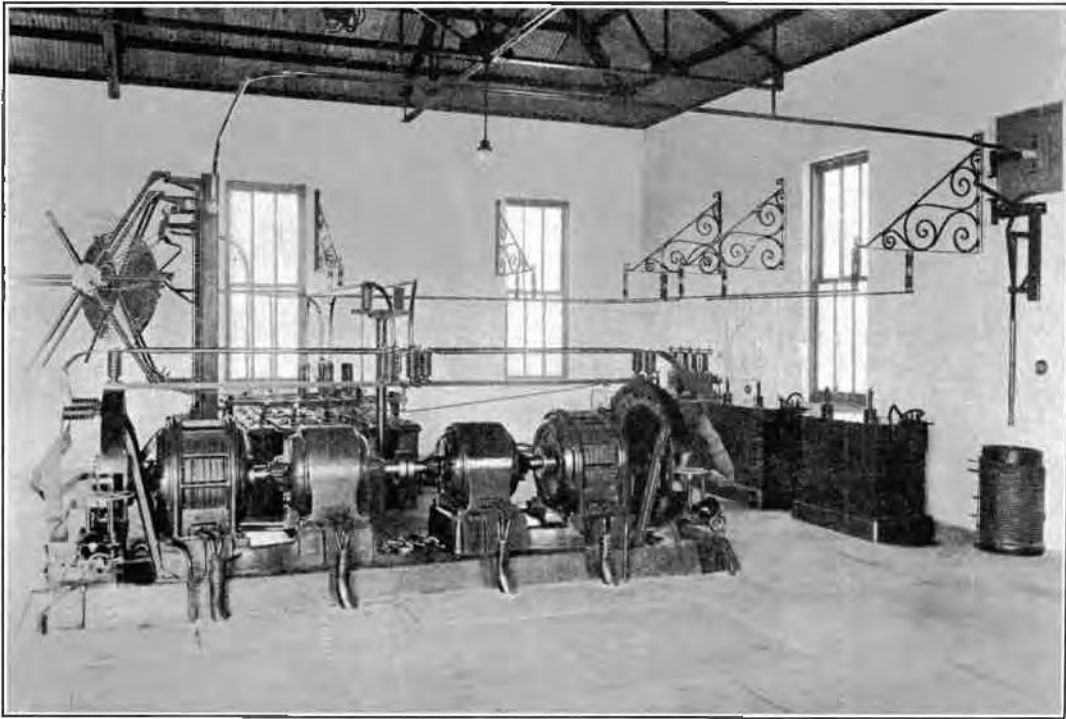
Power Plant of the New Orleans Station of the Tropical Radio Telegraph Company, showing the 50 K.W. Transmitter
